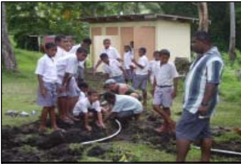
The new pipes being laid in the school grounds under the watchful eye of head teacher
