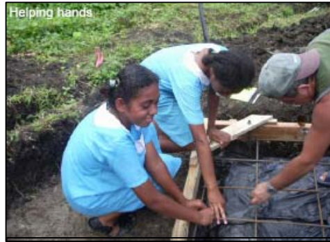
School children assisting with laying a concrete base for the SkyHydrant Safe Water shelter
