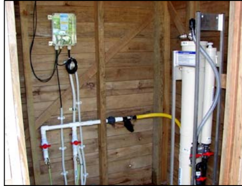
Contaminated water from the mountain stream is gravity fed under low pressure through the SkyHydrant water filter to produce safe potable water. The water is then pumped to two tap stands for easy access for the school children
