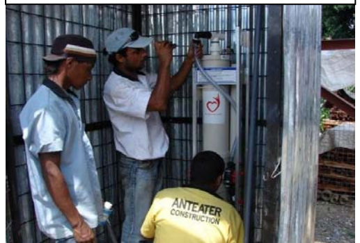
Water management committee commissioning the SkyHydrant in the protective steel enclosure
