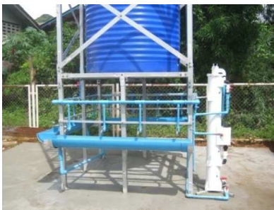
Back view of the water system
