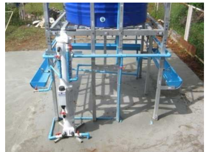
Front view of the water system
