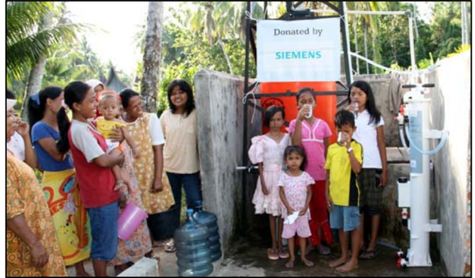
Families bring their 20 litre water containers to be filled with safe water from the SkyHydrant
