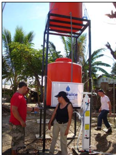
The completed SkyHydrant system in Bairo Pite Clinic - Dili
