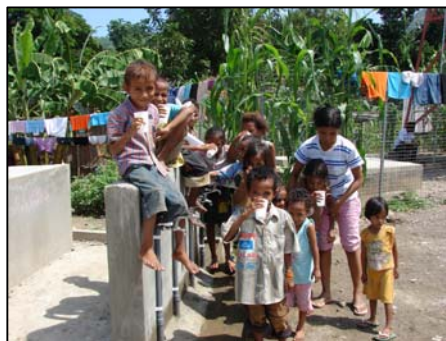
Since the installation of the SkyHydrant water treatment unit, water tankers are no longer required for the IDP camp, saving thousands of dollars per month
