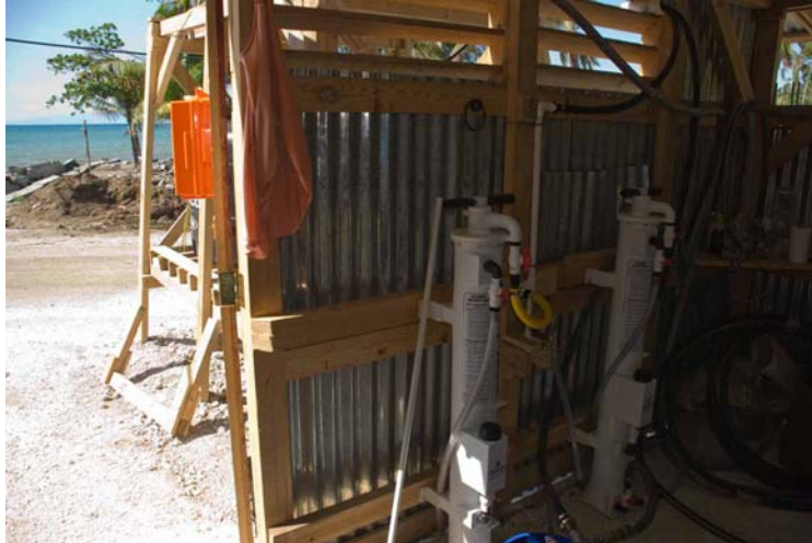
Two SkyHydrants installed at the main site in Petit Guinée
