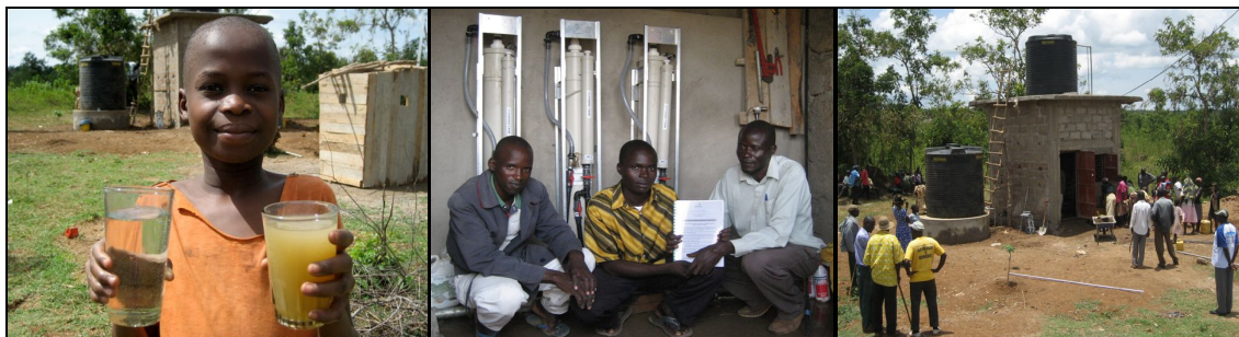
Figure 4: Kenya Safe Water Kiosk Obambo-Kadenge Village installation which includes wind power and three units.
