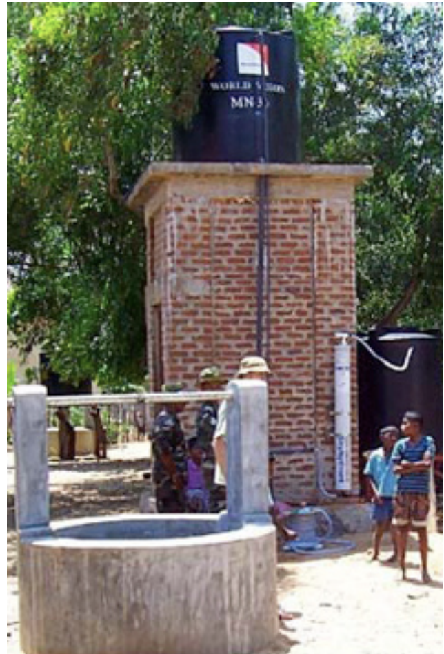
Skyhydrant Installation - Membrane module is mounted vertically on the side of the building
